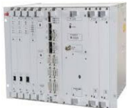
Communication Equipment (Power Grid)
