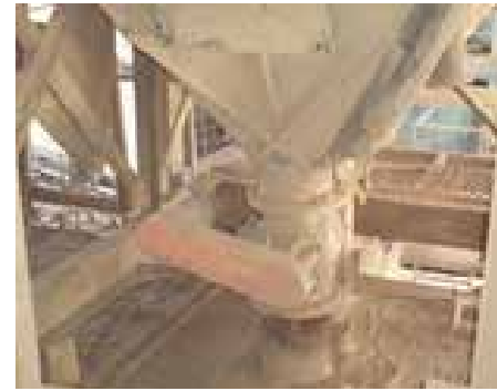
Replacement of New DC Bag Hopper Rotary valve in SSP of Production belt
