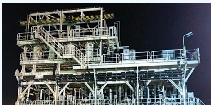
Barge mounted High Purity water system for Reinjection for an oil major in UAE
