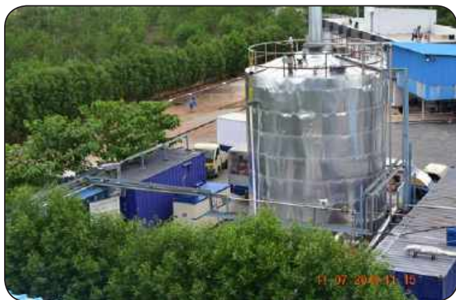
ANDICOS Waste to Energy Plant
