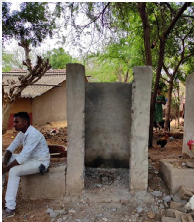
Toilet before Renovation
