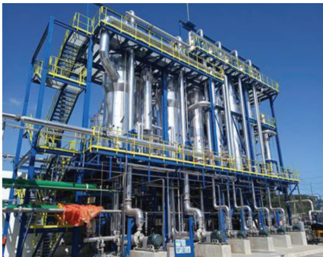
Praj successfully handed over a biometanated vinasse pre-treatment & evaporation plant, & modernized distillery plant in Dominican Republic.
