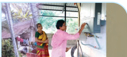
Setting up of a Solar Power Plant for 'The Goa Hindu Association Sneha Mandir' the old age home in Goa
