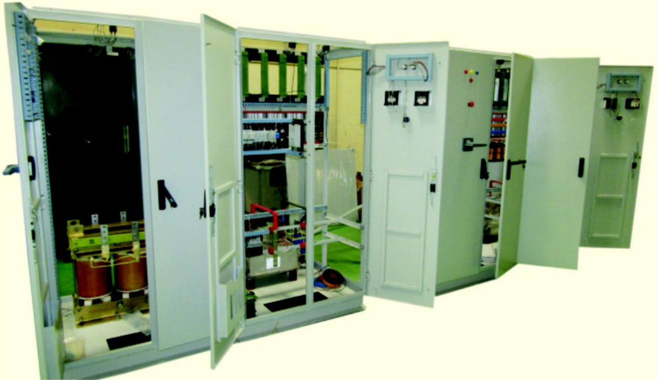
SUPPLY OF 1133V / 365A RECTIFIER FOR DC INJECTION BRAKING PROCESS
