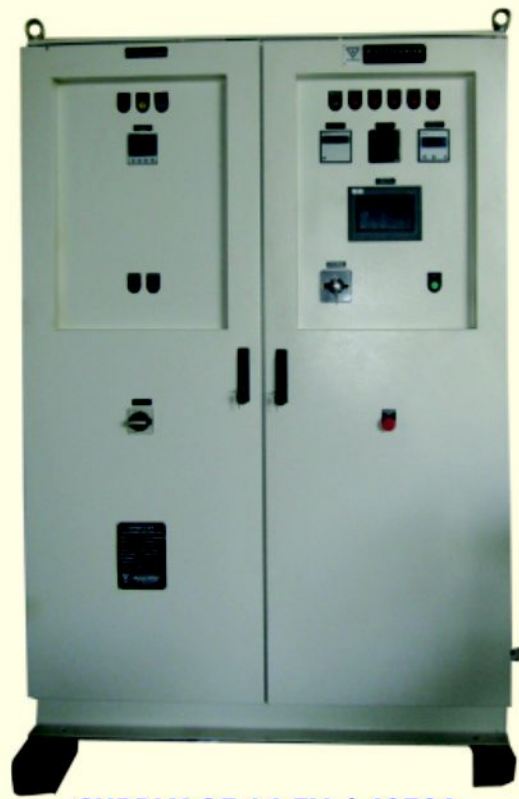
SUPPLY OF 14.5V / 4050A PRIMARY SCR CONTROL RECTIFIER FOR HYDROGENATION PROCESS
