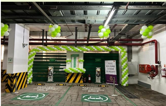
EV Charging station installed at Birla Aurora
