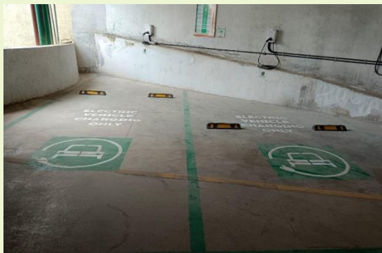
EV Charging station installed at Birla Centurion
