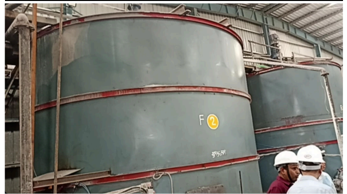
Fig 2 – Ash and water slurry storage tanks
